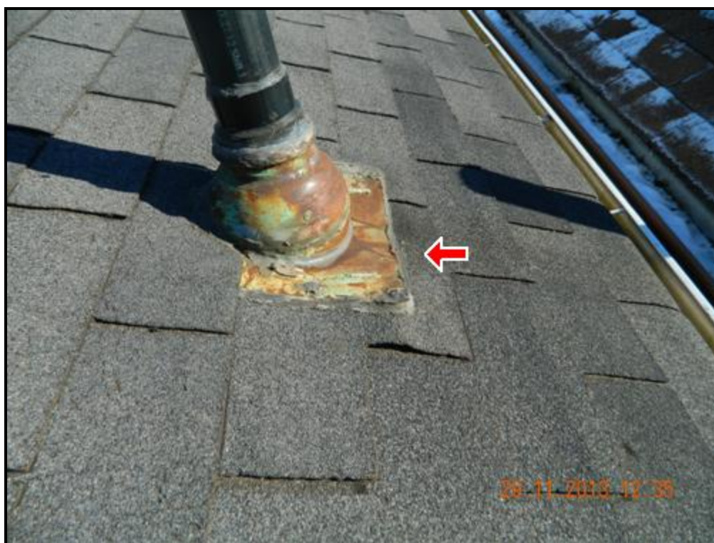
3.2 Picture 2 PLUMING VENT VIEW
